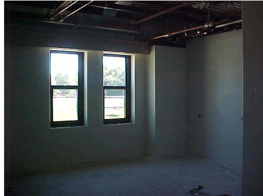
Windows in classroom
